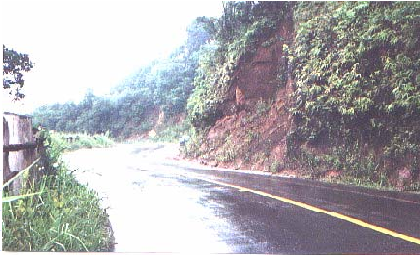
Figure 8 - environmental damage in a cut slope due to failure of the soil mass.
