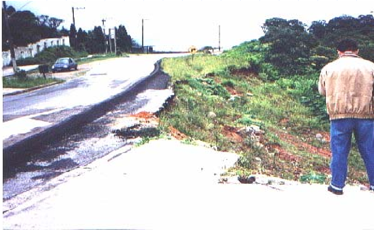
Figure 6 - earth fill failed at the entrance of the city.
