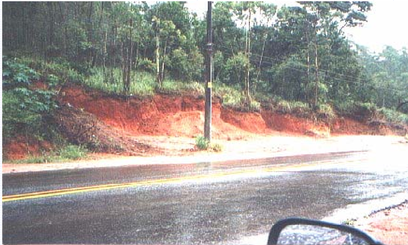
Figure 10 - borrowing area with erosion and instable cut slope.
