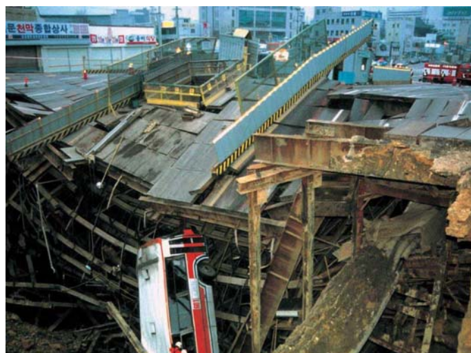
Figura 10 – Colapso del Metro de Taegu ( cut and cover ), Corea del Sur, 2000
